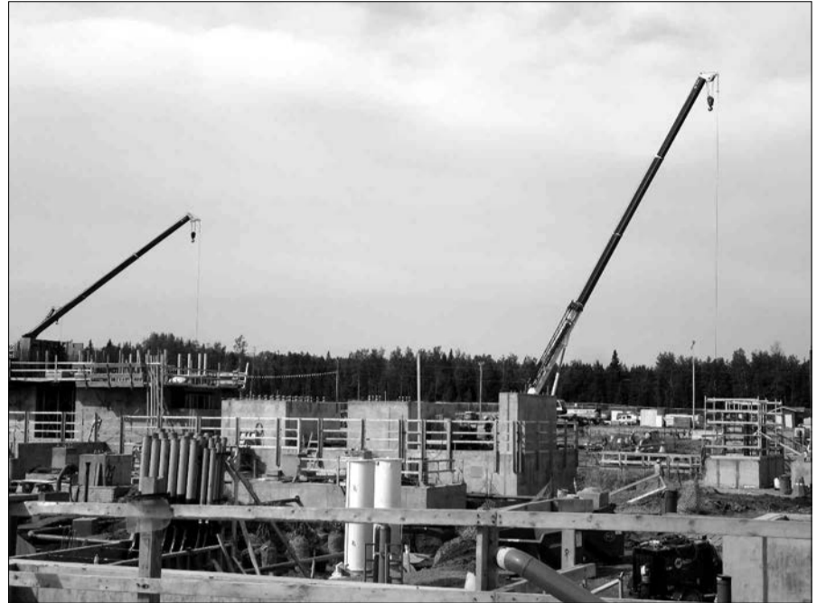
The Cascade Power Plant has a lot of work going on 24 hours/day. With an expected project completion in 2023, the $1.5 billion dollar 900-megawatt facility will power 900,000 Albertan homes. photo Shaylyn Thornton
