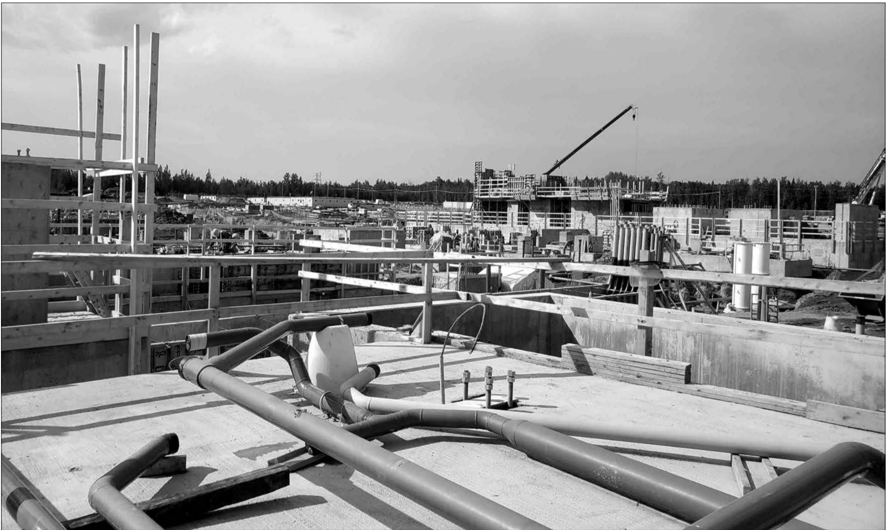
The crane in the distance is just one of many cranes and pieces of equipment being used to construct the Cascade Power Plant. photo Shaylyn Thornton
