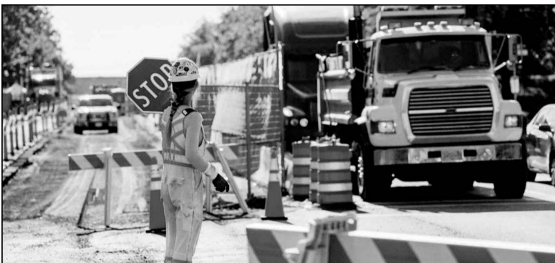
Variable Speed Corridors: Between Yellowhead Highway and Hope you may encounter a few variable speed corridors during a road trip. There are three, 20-minute intervals totaling a possible 60 minutes of delays on this trip, for the entire length of the highway corridor. This is monitored through TransMountain's extensive traffic management program.
