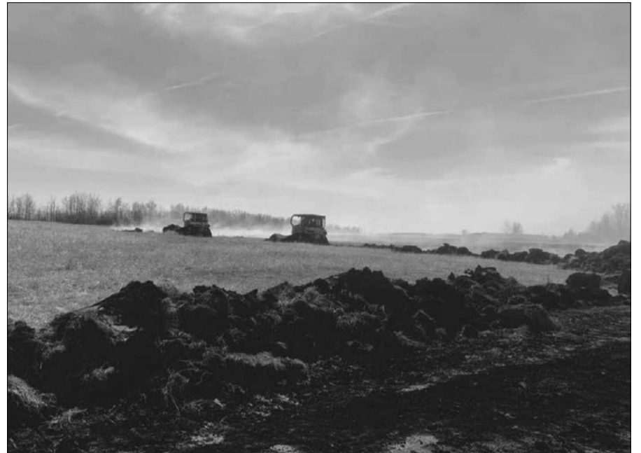
Dozers assisted with building containment lines around the perimeter of WCU002 (May 1, 2023 at 7:00 p.m.).
