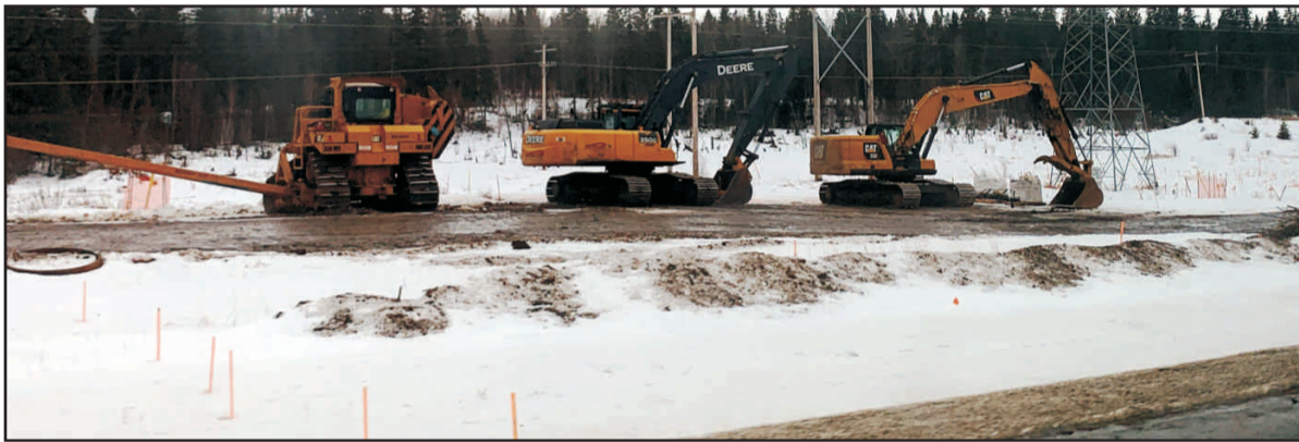
Work continues on the Trans Mountain Pipeline through Yellowhead County. Construction is taking place in a series of phased events extending west along the Yellowhead Highway past Hinton. photo Joshua McArthur
