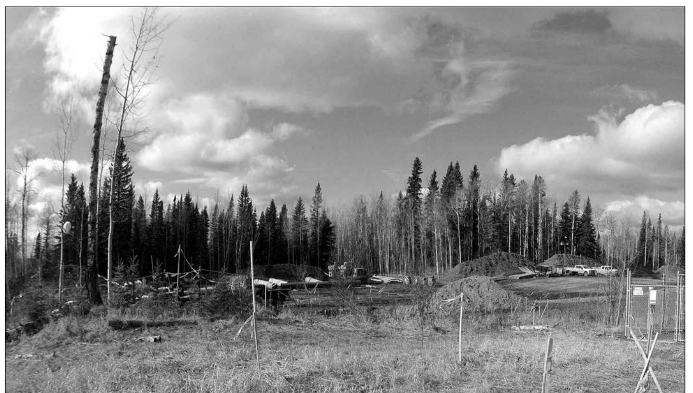
Work continues to progress on the Trans Mountain Pipeline 17 kilometres west of Edson near Bikerdike. photo Paul Kindiak
